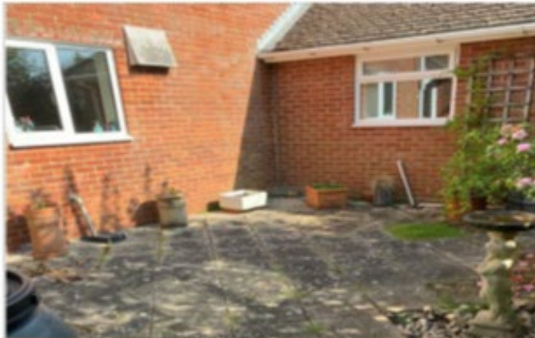
Fig. 1: View looking roughly north with Hangerfield's kitchen window to the left, and en-suite bathroom window to the right (not a part of grounds for objection).
